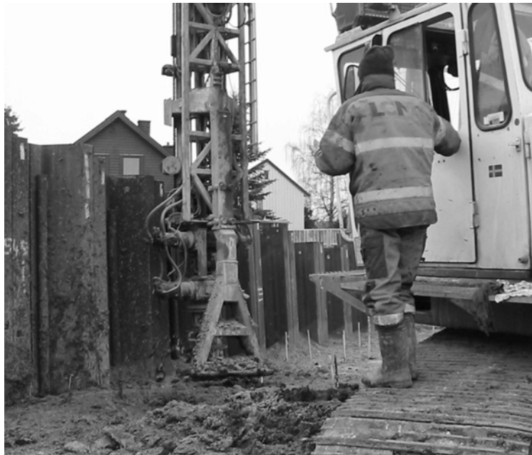
Figure 7: Installation of LCM Columns for passive support on a sheet pile wall in Asker, Norway.
