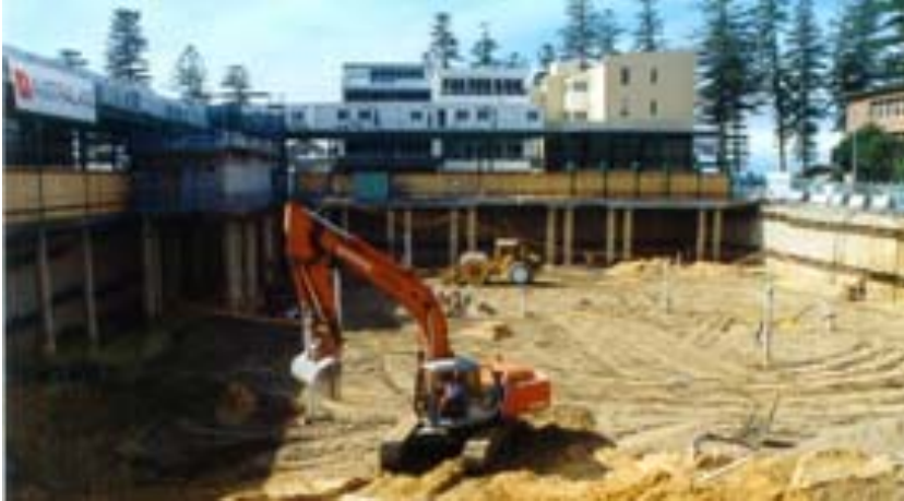
Figure 1: Densification to increase the bearing capacity and reduce settlement in marine sand.
