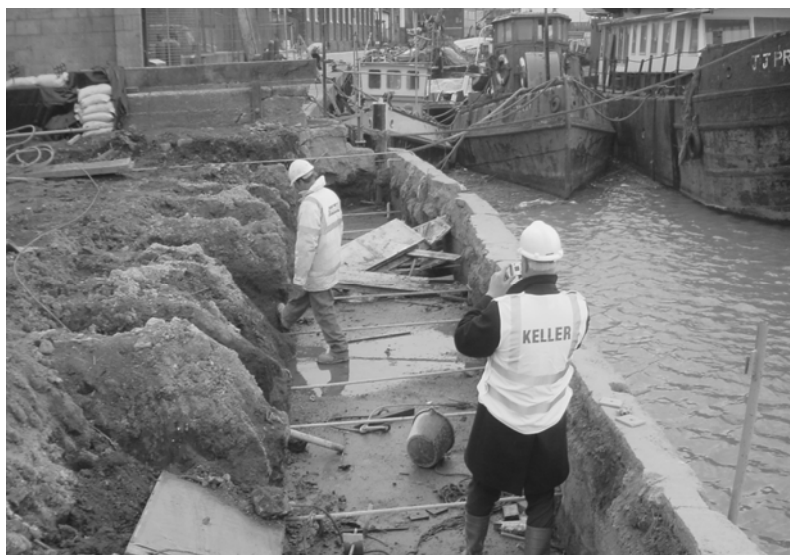
Figure 8: LCM mass gravity block behind existing quay wall at Barking, United Kingdom
