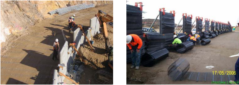
Figure 7: Reinforced soil wall installation using: (a) Inextensible reinforcement - Lane Cove tunnel project, Sydney, and (b) Extensible reinforcement - Tullamarine Calder Interchange, Melbourne.
