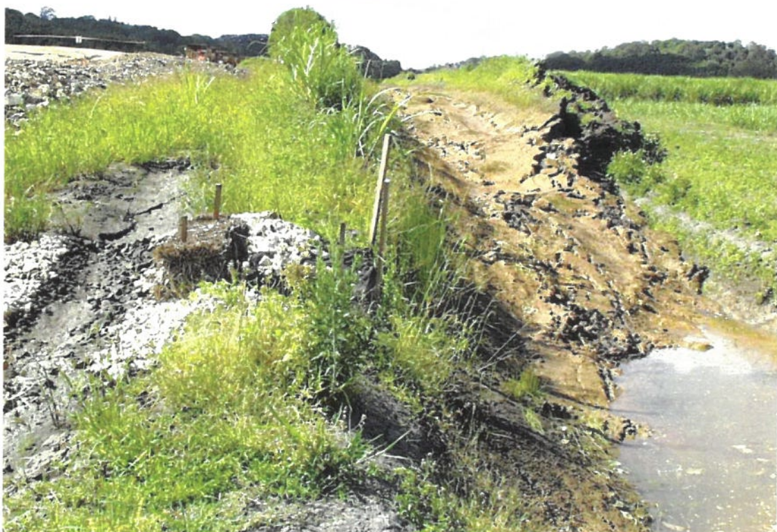
Figure 2: Ground heaving adjacent to toe of embankment
