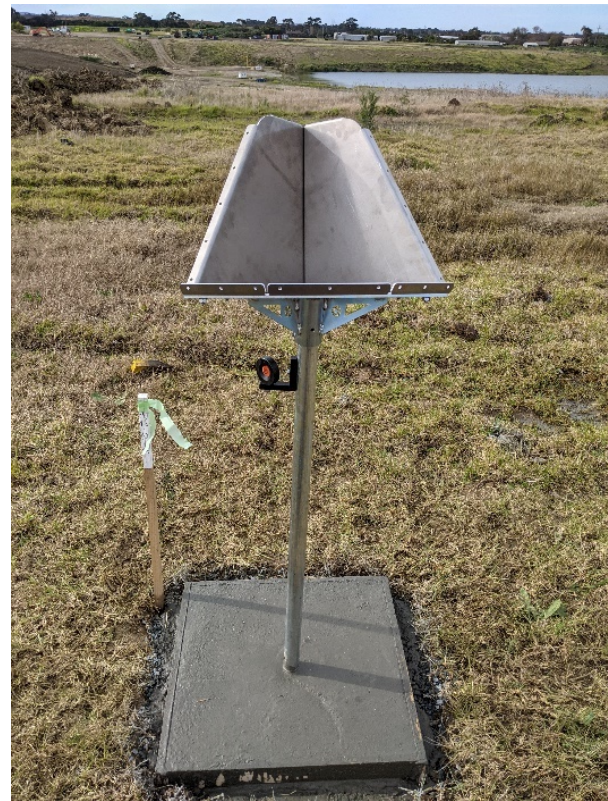
Figure 3. InSAR reflector installed at the SRL stabling yards (courtesy of Sixense Oceania).
