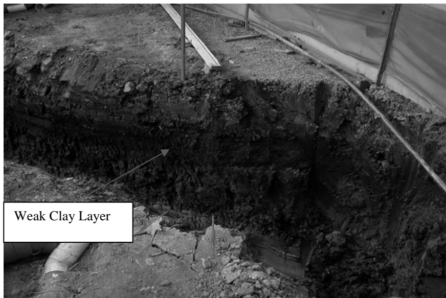
Figure 15: Excavation to East of Unit showing weak Clay layer.
