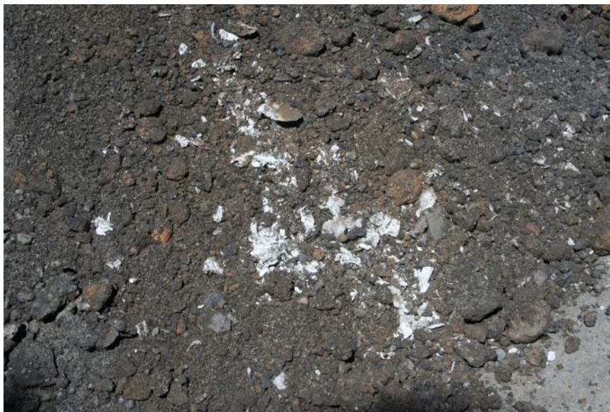
Figure 3: Degraded fibrous cement sheeting with asbestos in contaminated railway ballast.
