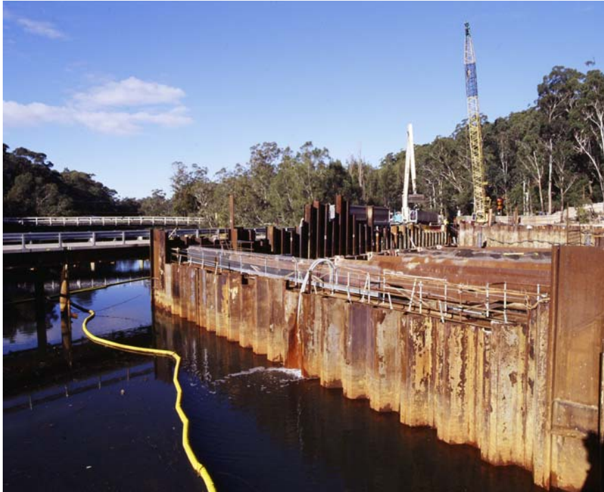
Figure 2: Acid sulfate soils being removed from the ECRL western cofferdam, Lane Cove River, NSW.
