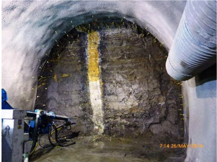
Figure 5: 800mm wide dyke in tunnel face.
