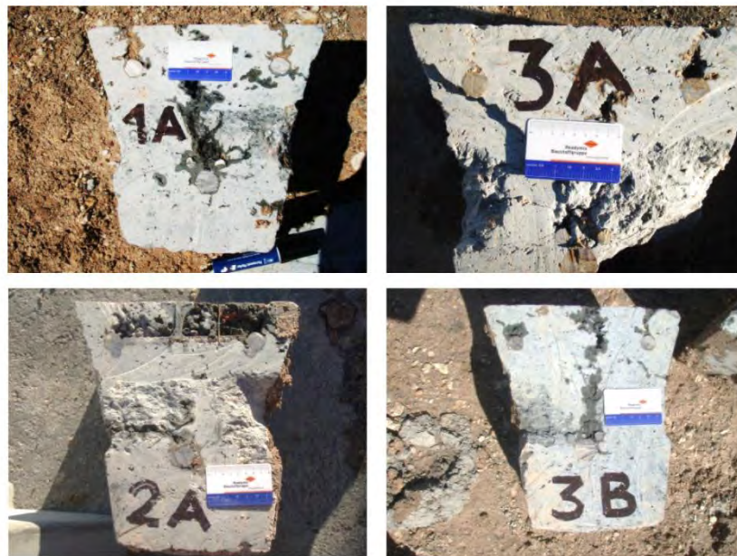
Figure 4: Evidence of shadowing of shotcrete (when used with accelerator) around steel lattice girders.
