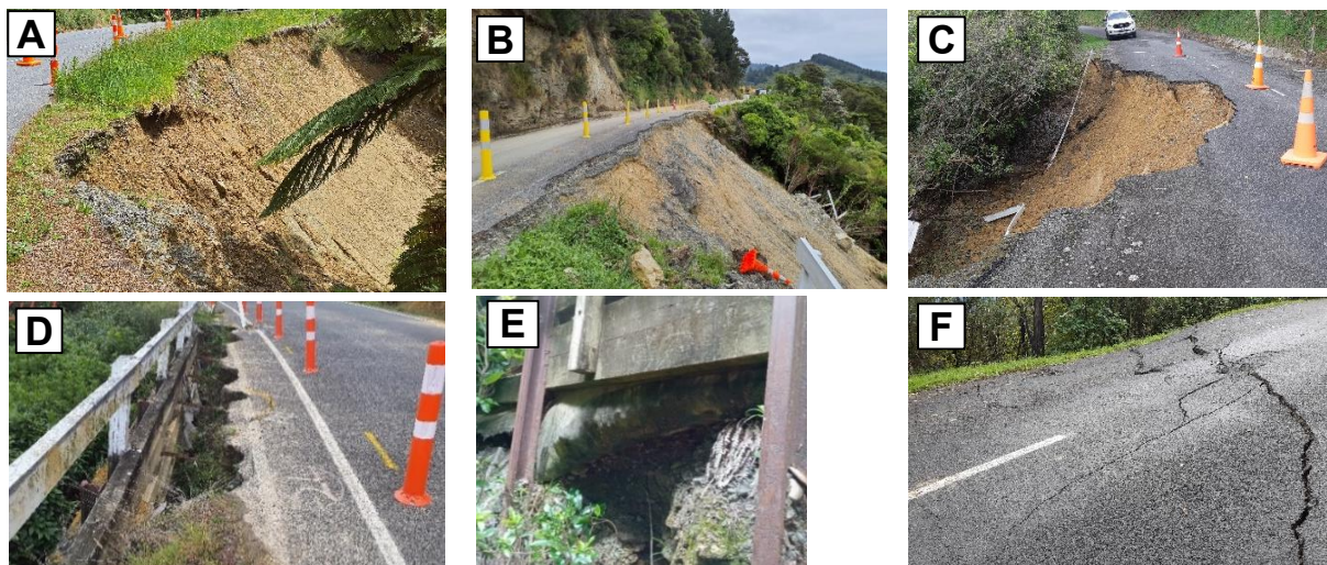
Figure 3. Typical examples of underslips and wall failures. (A) Planar soil slide. (B) Side-cast fill failure into a planar slide. (C) Rotational slide at MBR RP3.0. (D) Void behind rail iron retaining wall. (E) Loss of backfill below lagging. (F) Global slope deformation.
