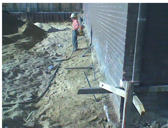
Figure 6: Permeation grouting to limit settlement due to sheet piling at Woolworths Umina
