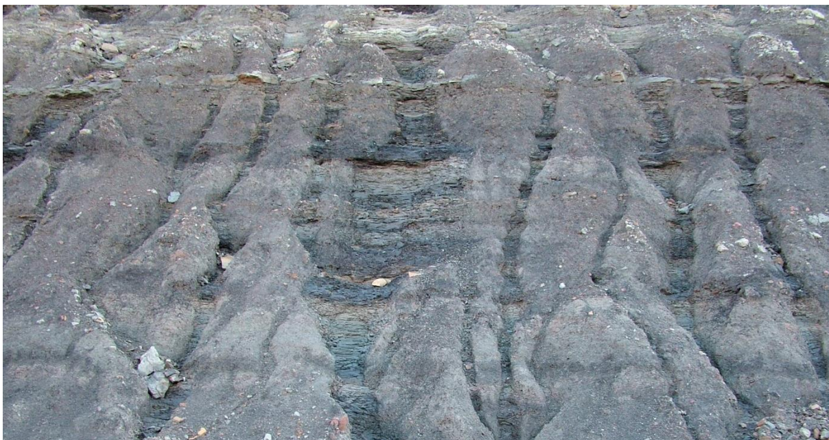
Figure 3: Rock mass degradation on exposure in quarried batter
