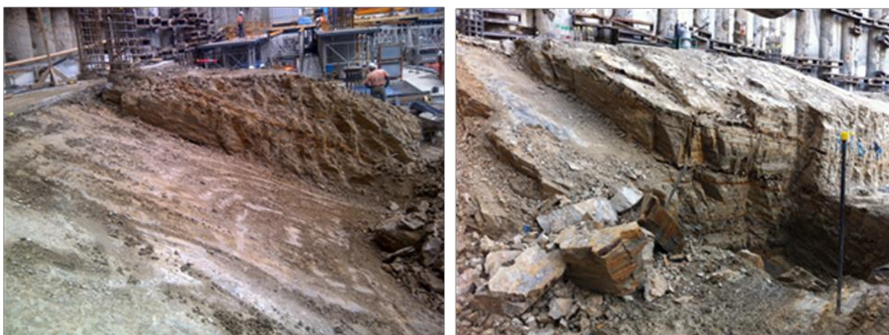
Figure 1: Photograph showing a slickensided bedding plane which caused movement of the retention system of the east wall of the excavation in excess of design
