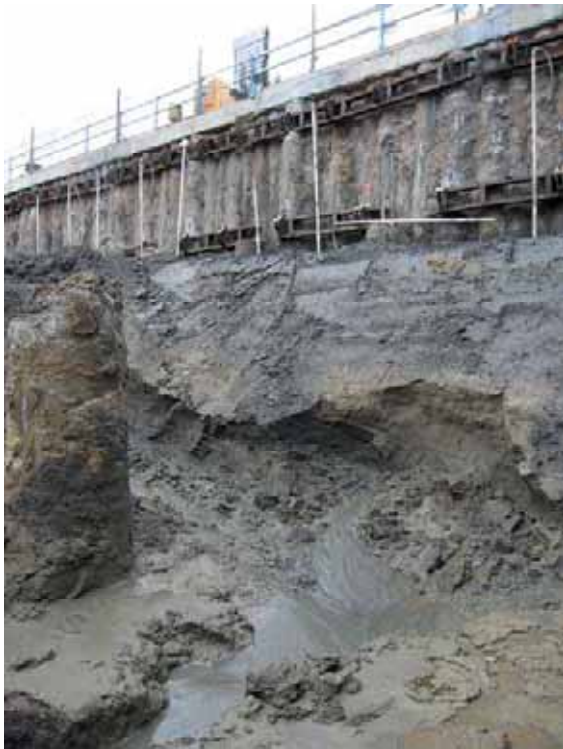
Figure 3. Water flow into basement excavation
