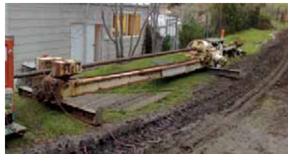
Figure 7 - The drilling rig mast separated from the drilling rig
