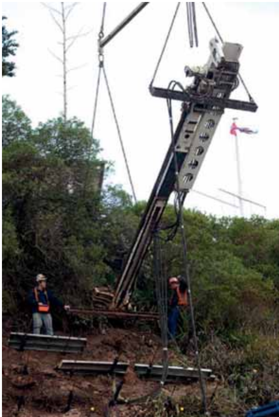
Figure 12 - Soil nail installation on the upper section of the slope. Note; driller operating the remote controlled rig on the left.
