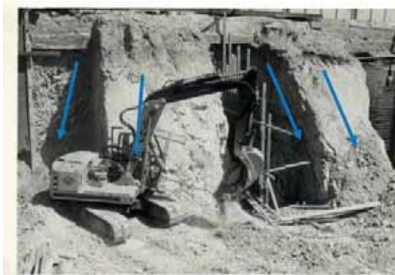
Figure 4 Trench excavations for footings adjacent to the southern boundary to maintain external support to the adjacent ground and structures. A completed footing and wall with starter bars can be seen on the right of the image. The inferred typical rock dip direction is indicated.
