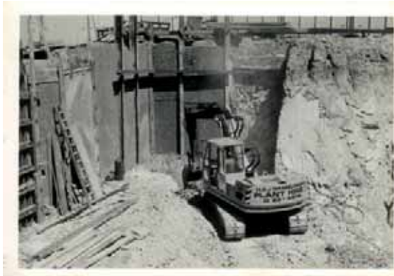
Figure 3 Original basement excavation showing the 250UB channels as part of the temporary works.
