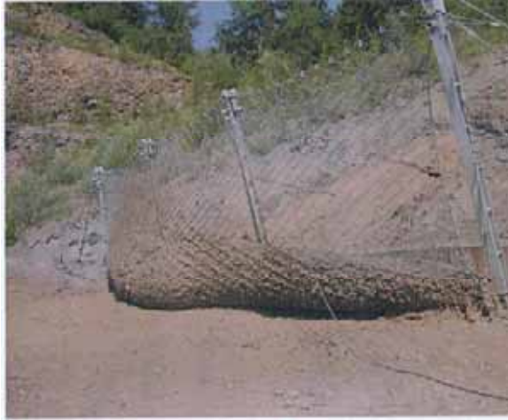
Figure 10. Debris Flow Barrier (Geobrugg)
