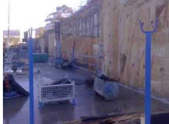
Figure 6. Example of Face Cut with Diamond Saw Fitted to Excavator, Rock Bolts in Place
