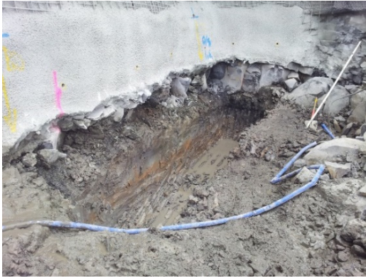
Figure 9: Contact between basalt and Tauranga Group Alluvium exposed in short sections prior to concrete mass block stabilisation. Note the stiff nature of the soils evident by the stability of the vertical cut.
