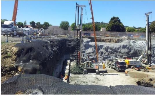
Figure 7: Continuous Flight Auger (CFA) piling rigs forming the stabilised block behind the tunnel portal headwall.
