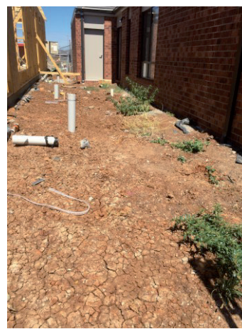
Unsealed building perimeter with reverse slope towards footings. No stormwater collection or diversion. (Note soil cracking indicating highly reactive clays present.)
