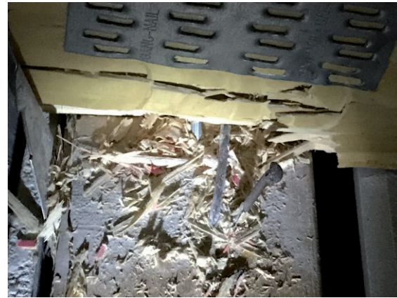
Figure 6. Fractured truss chord at a tie-down to internal wall.
