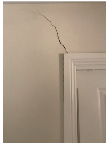
Figure 1. Example of a “slight” (category 2) crack to AS2870 (noting that plasterboard is rarely articulated).
