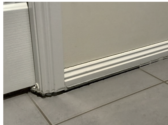
Figure 7. Internal stud wall attached to roof trusses, entirely lifting off floor slab due to edge heave.
