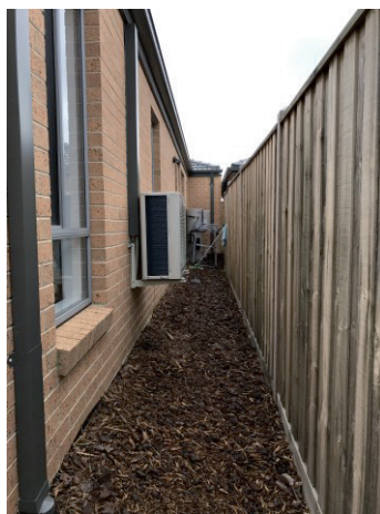
Unsealed building perimeter with no collection and sub-surface discharge of stormwater. Permeable “tan-bark” landscaping.
