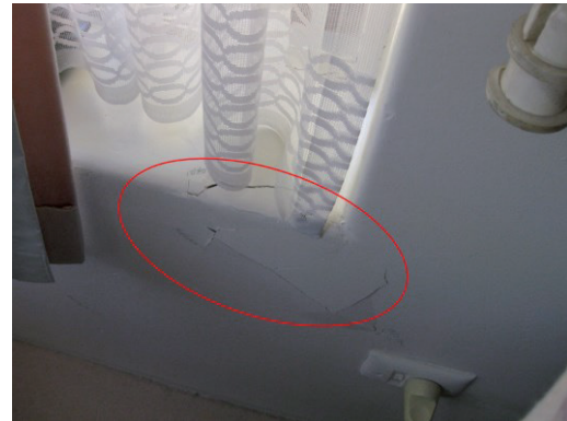
Figure 11. Cracking on the wall of bedroom
