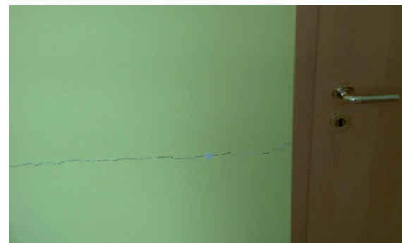
Figure 1. Example of a horizontal building crack caused by foundation soil swelling in a residential building
