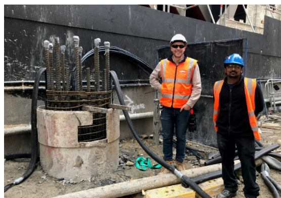
Figure 4. An energy soldier pile wall trial in Melbourne helps learning by doing and helps quantifying real (as opposed to perceived) risks associated with the technology.
