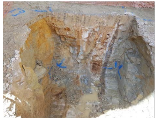
Figure 7. Spread footing (base not yet cleaned) with exposed weaker dyke material in base and sidewall
