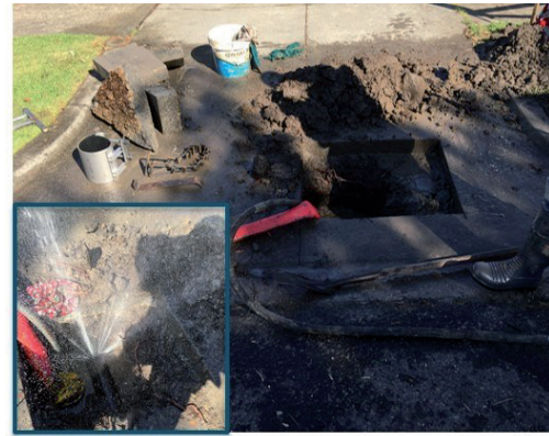
Figure 6. An example of failure for drying under driveways; failure is at centre of driveway
