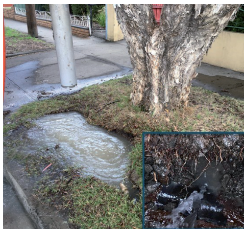
Figure 9. Example failure near tree roots
