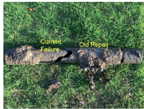
Figure 10. Example failure at a possible leak
