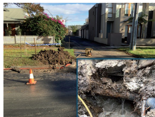
Figure 7. Example of failure for wetting under driveways; failure is at driveway edge
