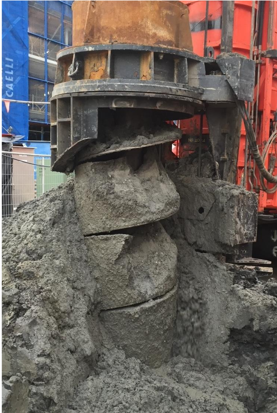
Spoil on Auger (Heavily transported)
