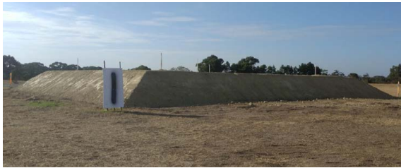
Figure 2. An example of a surcharge trial pad constructed to help assess settlement rates
