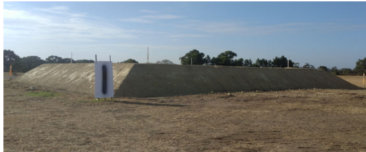
Figure 2. An example of a surcharge trial pad constructed to help assess settlement rates
