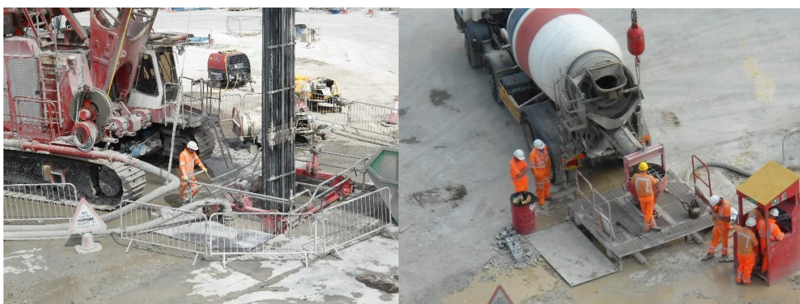
Figure 7: Edge protection barriers fixed to guide walls (left) and panel covers during concreting (right)
