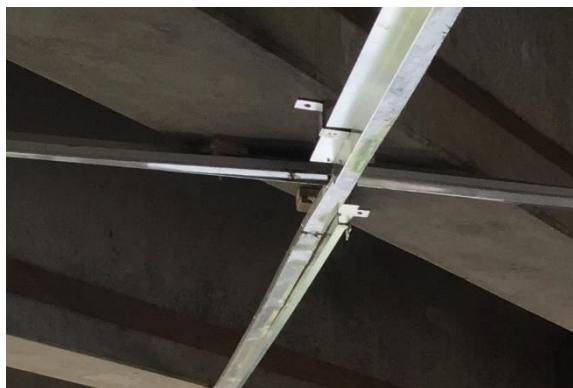
Figure 6: Diagonal Sensor Cable Ducting Attached Using Aluminium Angle
