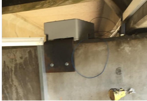
Figure 7: Junction Box Fitted Over Headstock Clamps
