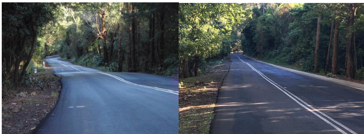
Figure 12: The image on the left shows obvious undulations on Mt Keira Rd at site 229 in 2012 (WCC, 2012) whilst on the right image the undulations are beginning to return in August 2017, 6 years after the work
