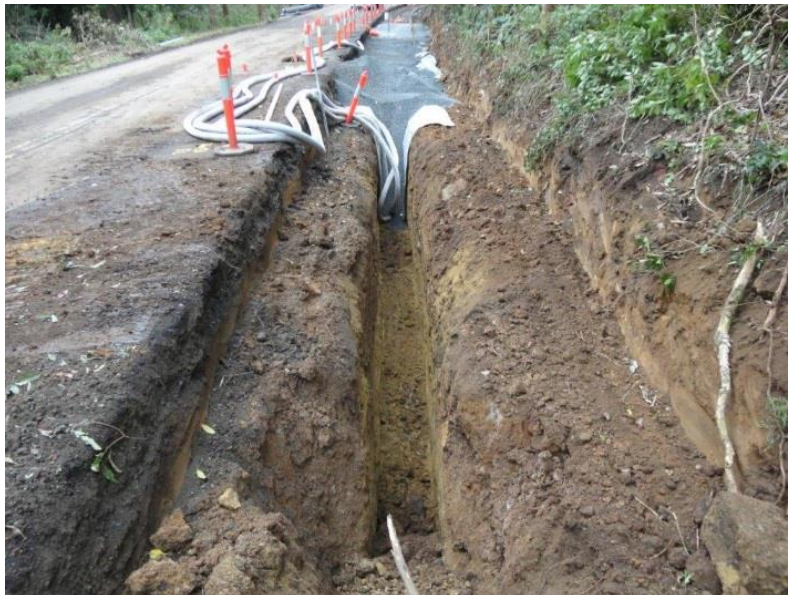
Figure 11: 2013 Excavation of a 4m deep cut-off drain along the road, with a concrete swale gutter above
