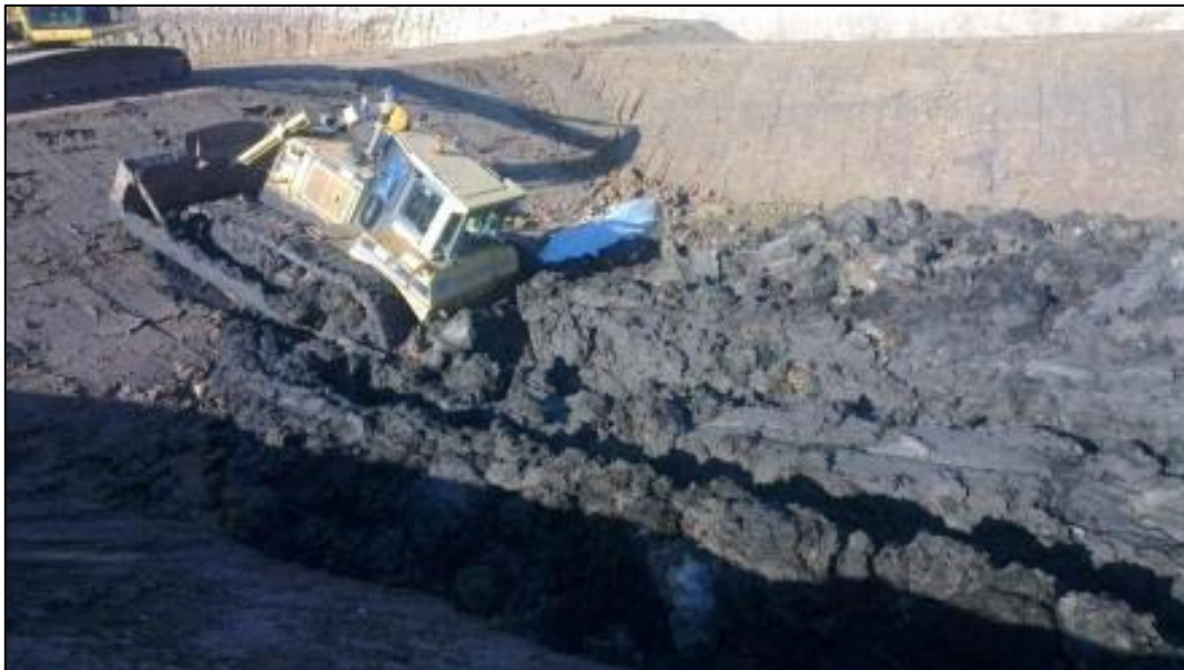
Photo 5: Unsuccessful attempt of swampy dozer to spread and compact untreated material within cell T1
