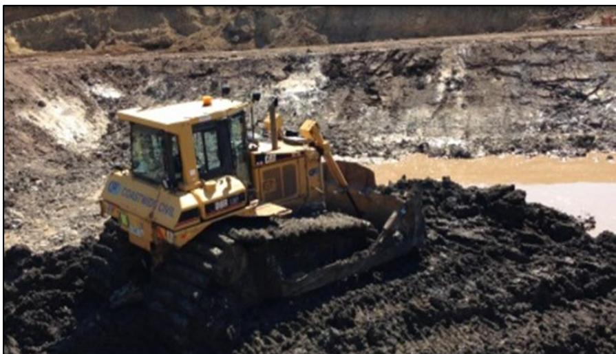
Photo 16: Swampy dozer successfully travelling on top of the first layer placed within cell T1 and treated by Hydrated lime
