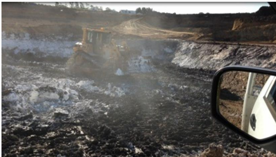
Photo 17: Swampy dozer successfully travelling on top of the second layer placed within cell T1 (treated by Hydrated lime) immediately after placement
