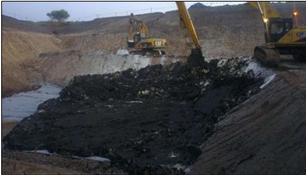
Photo 8: Long reach excavator mixing Aglime with ASSS material and then spreading and compacting it for the first layer placed within cell T2
