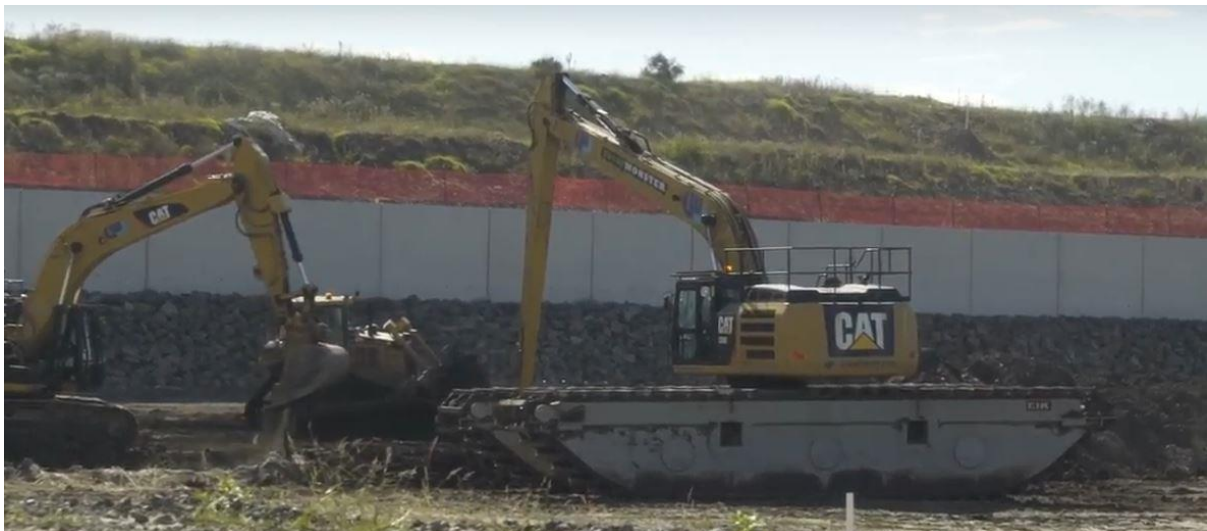
Photo 19: Picture of long reach excavator used by the Contractor with large, wide and long tracks used to track out over 'in the moist' ASSS untreated soils
