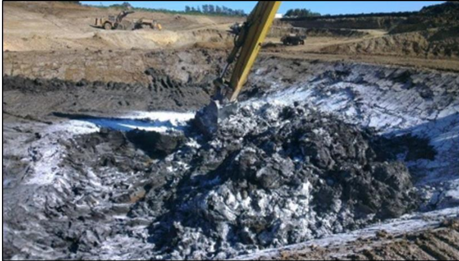
Photo 14: Long reach excavator mixing Hydrated lime with layer 1 of ASSS material within cell T1
