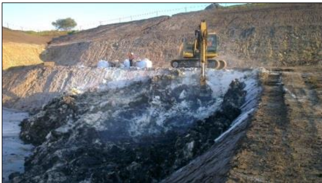
Photo 7: A small excavator spreading and mixing Aglime with ASSS material for the first layer placed within cell T2
