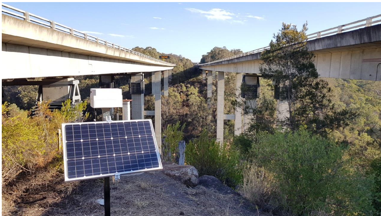
Figure 1: Low-cost Autonomous GNSS Monitoring Installation
