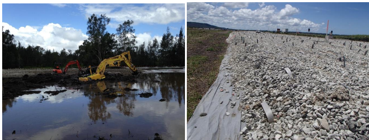
Figure 2: Early work construction on W2B (a) bogged excavator (b) wick drains installed
