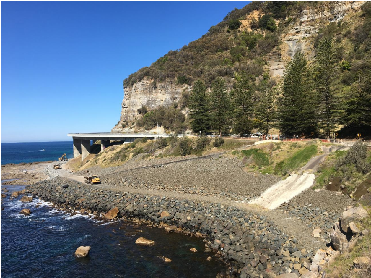
Figure 6: Slope showing rock revetment at the base of the slope, surface drainage measures and slope protection.
