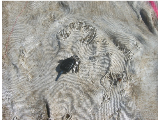
Figure 9: Typical high strength geotextile damage.
