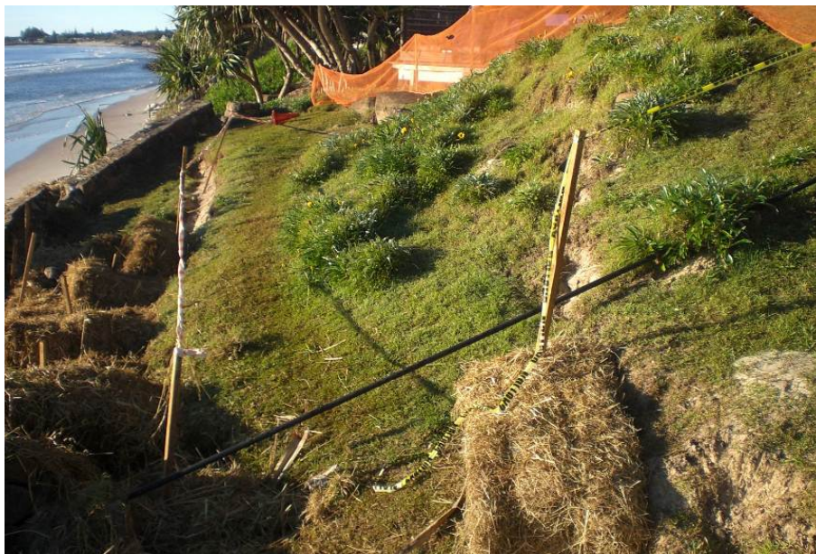
Figure 2: Tension cracks in foreshore slope indicating more deep seated rotational failures.
