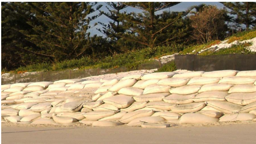
Figure 9: Sandbag revetment at Belongil Spit, Byron Bay, NSW 8 th June 2011 (photo courtesy Manly Hydraulics Laboratory)
