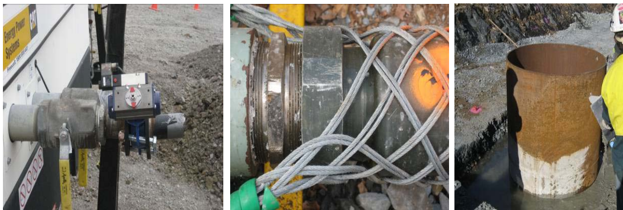
Figure 8: Automatic switch-off at compressor (left), typical whip check connection for high pressure air hoses (centre), casings should be installed as fall protection even if rock is close to surface (right)
