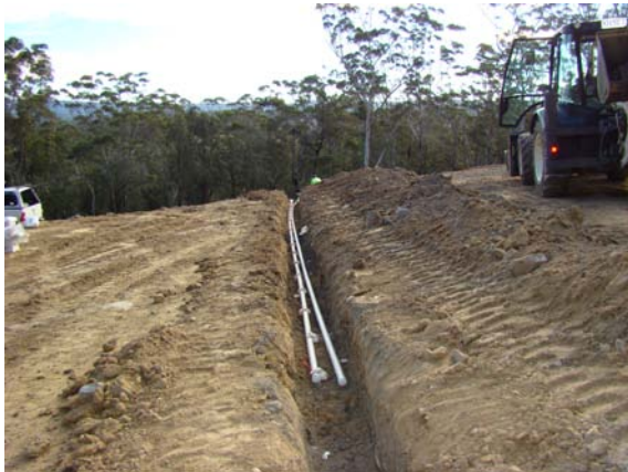
Figures 12: Monitoring trench PVC tubes for thermistor (right) and O 2 tubes with pink inlets (left).
