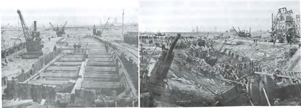
Figure 5: Pre and Post- cofferdam image, Alexandra Dock, Wales, July 1909 (Photo source: Jarvis, 2011).
