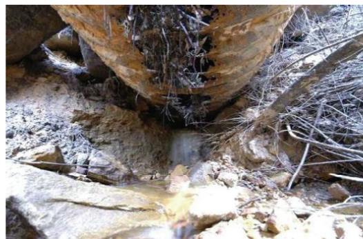
Figure 22: Perforation of pipe inverts at Leask Creek
