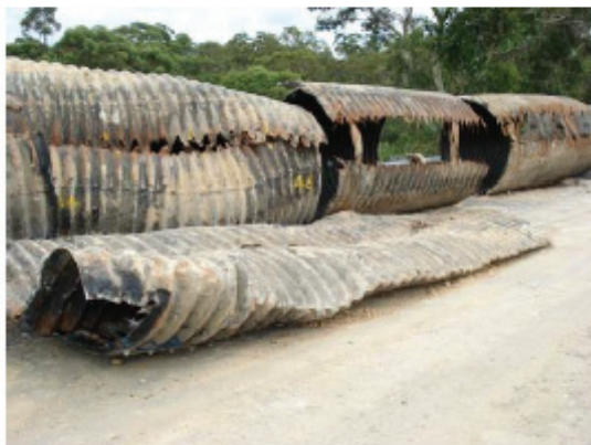
Figure 14: Deformation of pipe culverts
