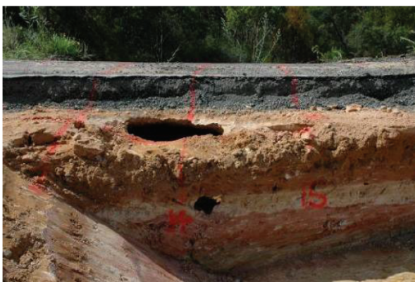
Figure 19: Voids in the embankment fill beneath the road Pavement
