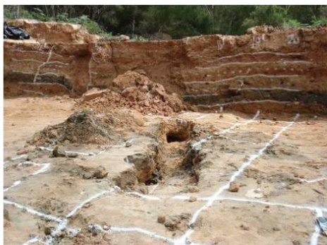
Figure 21: Further dipping of embankment layering and voids present above pipes
