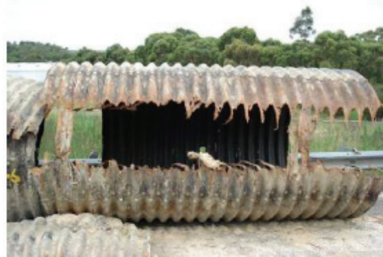
Figure 15: Perforation of pipe invert
