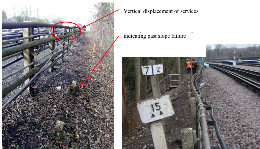
Figure 2: Signs of instability at crest: vertical displacement of services and partially buried cable (left photo) and leaning cable posts carrying cable runs (right photo).
