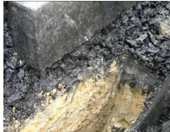
Figure 9: Ballast fouling due to coal and subgrade pumping (Goonyella System, QR National: Photo courtesy of Michael Martin)
