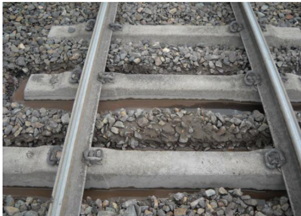
Figure 8: Mudholes caused by excessive coal/clay fouling (Goonyella System, QR National: Photo courtesy of Michael Martin)
