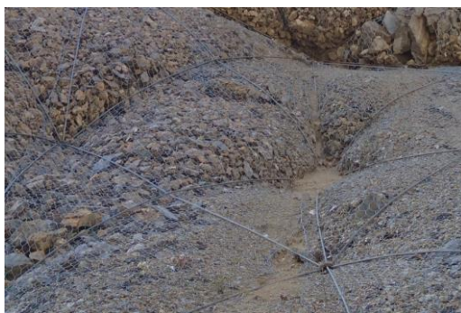
Figure 2: Large pockets of debris pushing on the facing and deforming the mesh.
