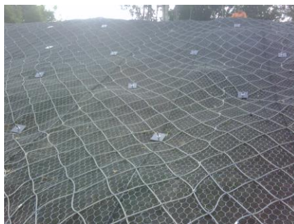
Figure 1: Soil nailing example of soil nailing with hexagonal mesh and steel rope panel or facing
