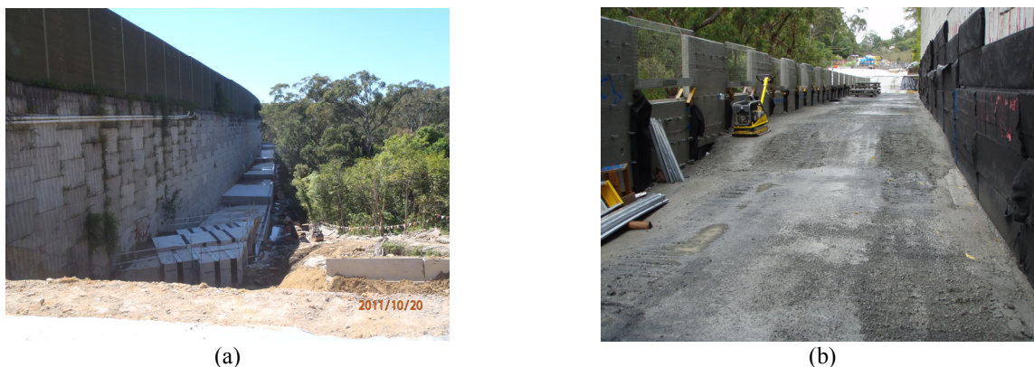
Figure 11: Construction of the CS-SRSW (a) Concrete platform completed (b) Initial layers of the stabilised DGB20 with details of the face panels and back double drainage system.
