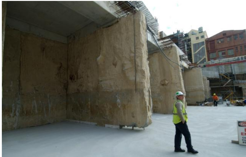
Figure 8: Application of temporary internal T panel buttresses at Perth's 100 St Georges Terrace tower
