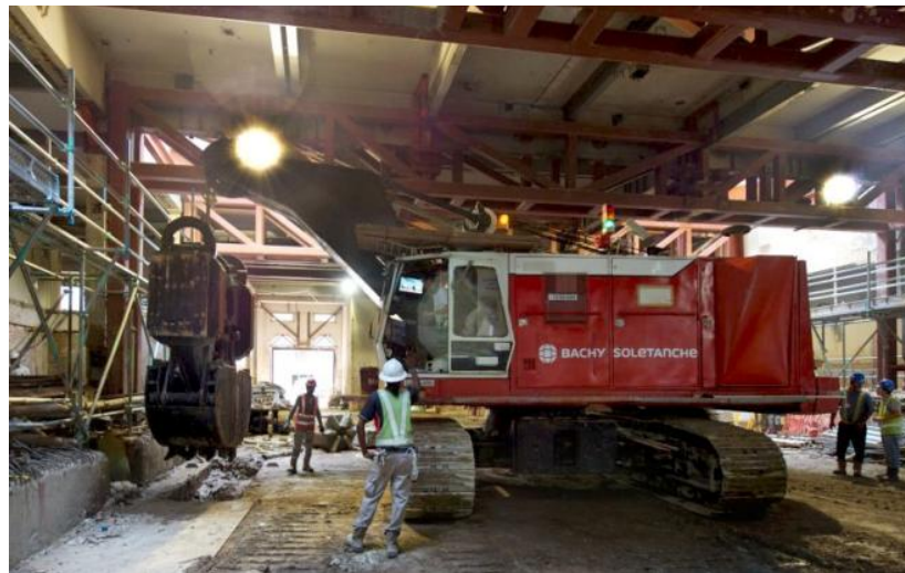
Figure 1: Specially designed low headroom excavation rig at work in a confined space of Singapore National Arts Gallery
