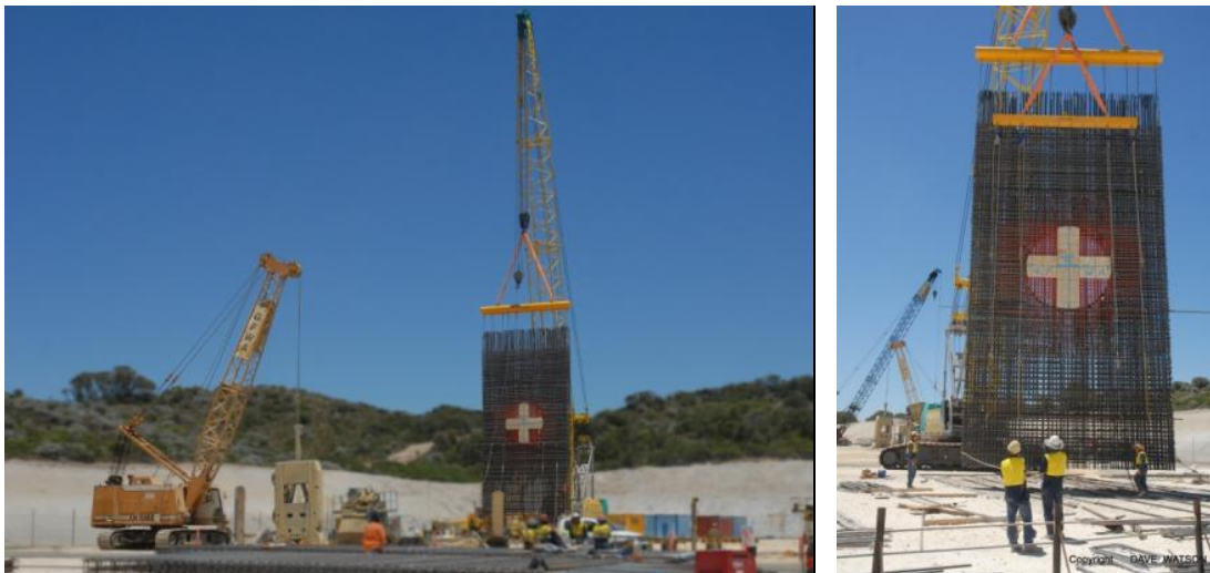
Figure 3: Implementation of glass fibre bars at Binningup Desalination Plant in Western Australia
