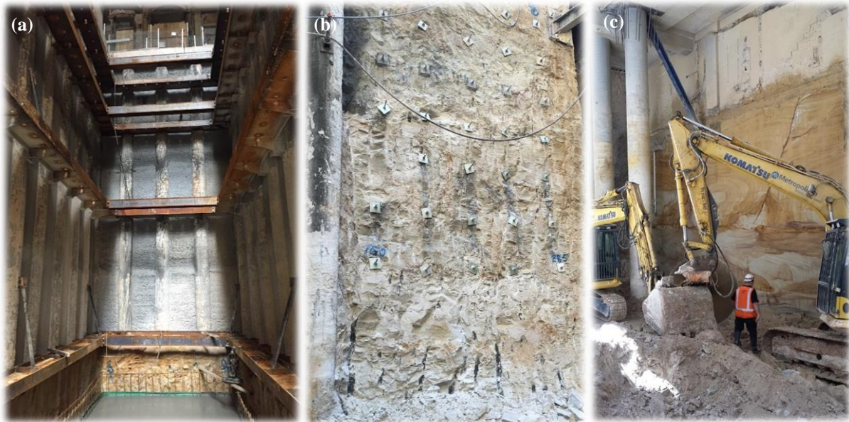
Figure 13: Details of the completed excavation: (a) vehicle lift shaft within GPO zone (b) zone of additional fracturing induced by the GPO fault (c) good quality sandstone on George Street side.
