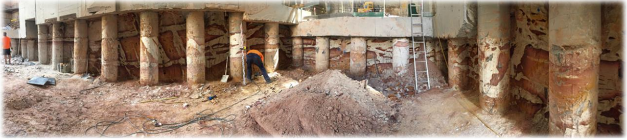
Figure 11: View of the first stage of excavation within the GPO fault zone.
