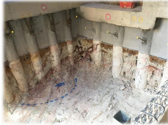
Figure 12: View of the second stage of excavation within the GPO fault zone.
