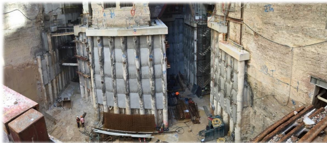
Figure 14: View of the completed excavation. Note: Spiden House on the left (with vehicle lift shaft), excavation around York Street heritage buildings, Carlton House on the right with zone of increased fracturing at the end of soldier pile wall.
