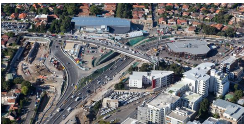
Figure 14: Extensive construction works at the proposed Concord Road Interchange in April 2017 (site photo).
