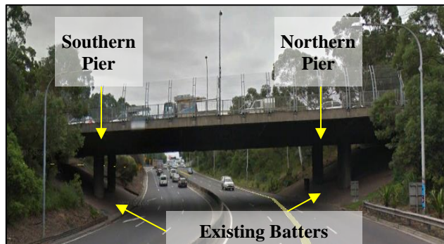
Figure 5: Elevation view of the existing Concord Road Bridge circa April 2016 (Google Earth, 2017)
