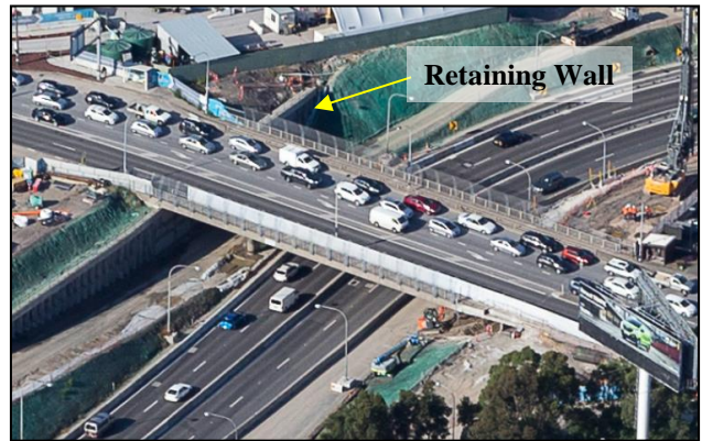
Figure 16: Cantilevered bored pile retaining wall along the northern side of the existing Concord Road Bridge in April 2017 (site photo).
