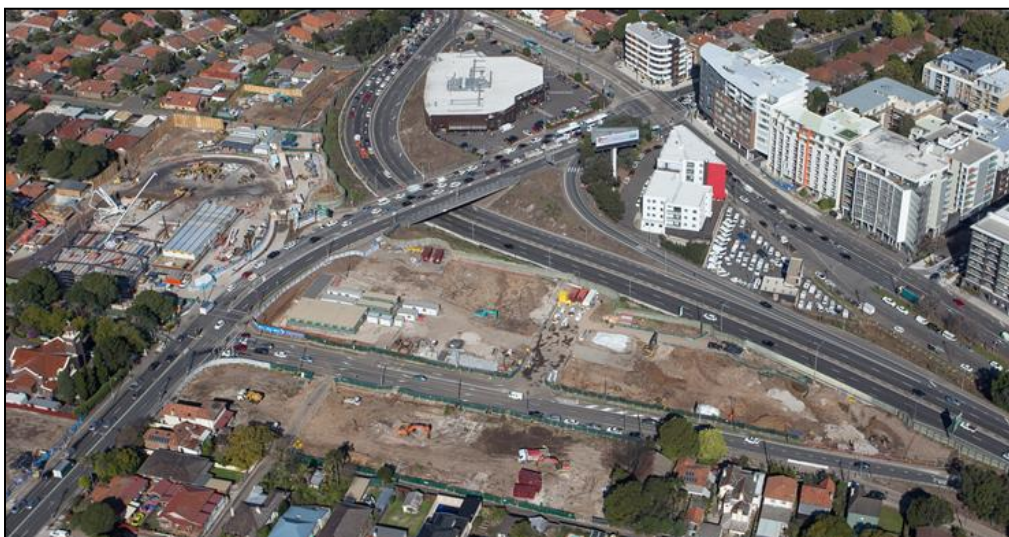
Figure 13: Construction works at the proposed Concord Road Interchange in December 2016 (site photo).
