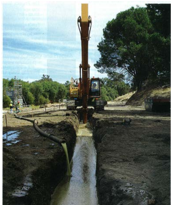
Picture 11: One of two parallel trenches dug to install permeable reactive barriers in Bellevue
