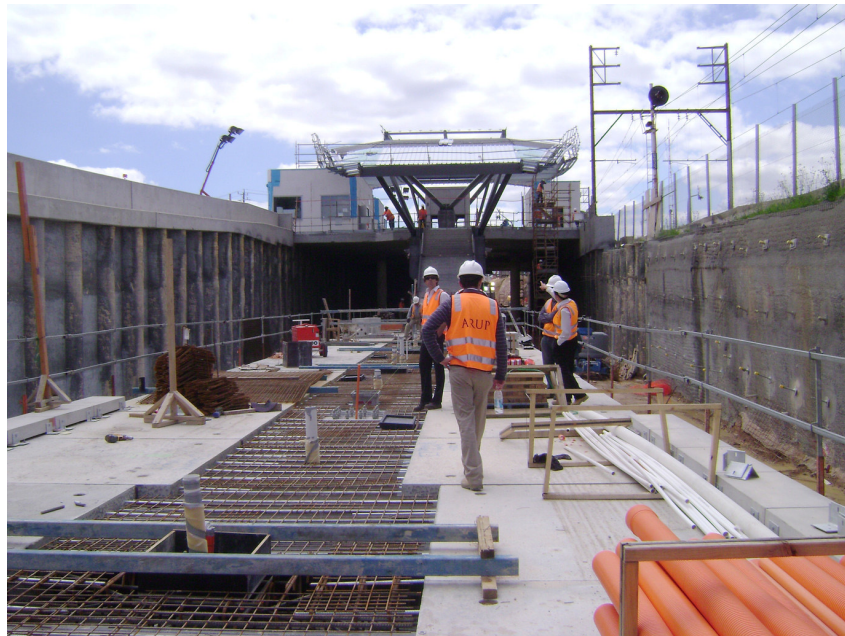
Figure 3: Embedded retaining wall (to left) with traffic barrier for road-rail grade separation in Victoria
