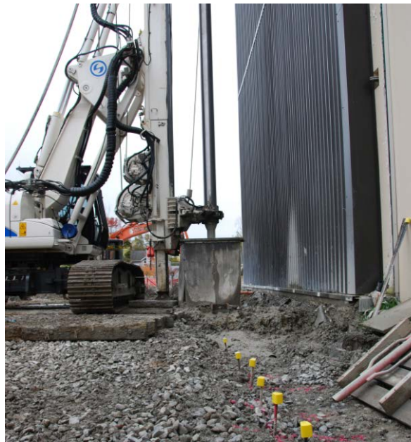
Figure 4. DSM installation in close proximity to an existing building with reduced vibration and noise compared with driven sheet pile or bored soldier pile options.
