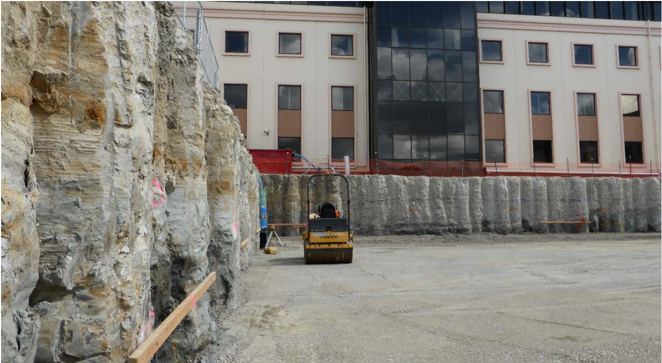
Figure 6. 4m deep basement excavation with typically dry walls with localised areas of dampness and no groundwater infiltration through the wall.
